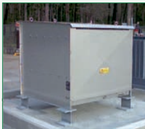
2*770 Ohm, 90s, 11.55 kV air cooled
